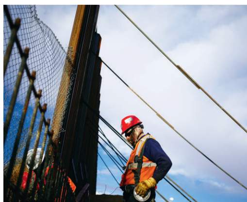
A section of a border fence separating the US and Mexico is under construction. Photo: Bloomberg
